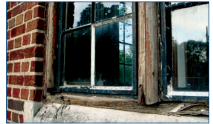
The windows at the Shelter are in bad condition.
